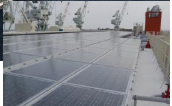
EMERALD ACE and installation of 160kW solar generation system on the deck
