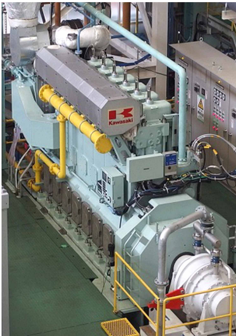
Gas-engine hybrid propulsion system
